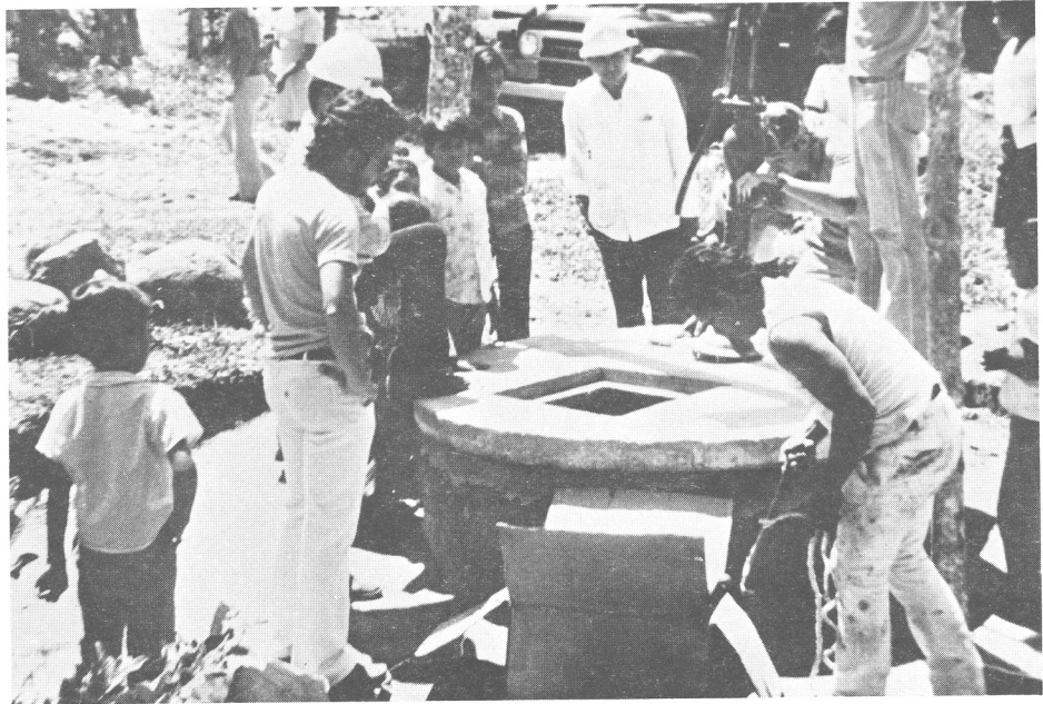
A hand-operated water pump is installed in LaGarita, Nicaragua with the assistance of the Engineering Extension Laboratory's Water Resources Group. The Water Resources Group has helped 11 underdeveloped countries to install and operate similar water pumps.
